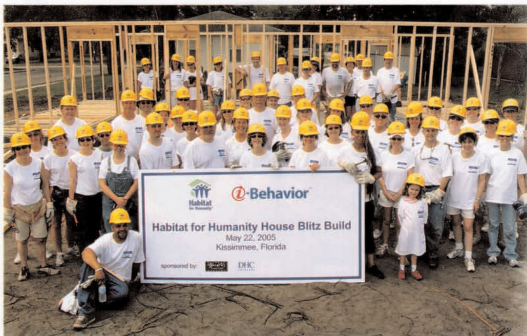
I-Behavior and 60 of its clients raised the walls of a Habitat for Humanity House as an alternative to the typical cocktail reception at trade show-related events.
