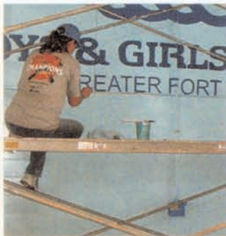
Timberland Co. and its clients paint the Boys & Girls Club's logo inside the building.
